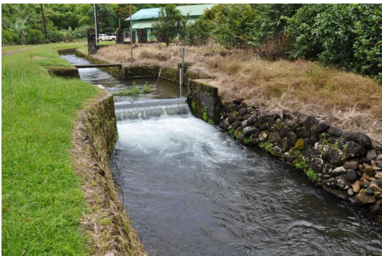
Photo: Water flows past the upper Waiahi hydroelectric plant
