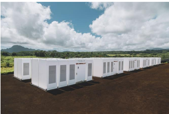
A total of 272 Tesla Powerpack lithium-ion batteries provide for 52 megawatt hours of solar dispatch during Kaua'i's evening peak
